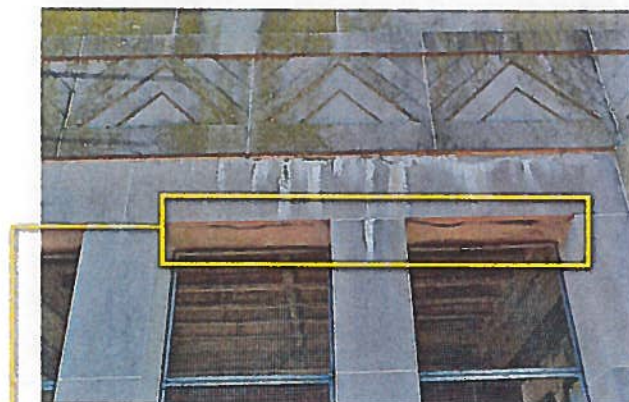
The framework around the openings at the top is eroding significantly. Screens are broken, and the area is accessible to birds.
